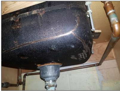
Asbestos-containing black mastic on the underside of sinks.
