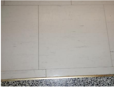
12" x 12" white with fine black streak pattern, vinyl floor tile with asbestos-containing mastic, present in Classroom 115.
