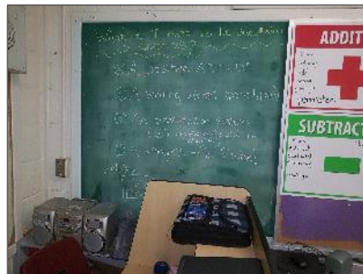
Presumed asbestos-containing Transite chalkboard.
