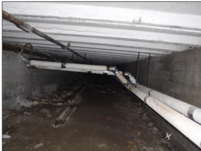
Asbestos-containing Aircell pipe insulation in the tunnel beneath corridor 116H.
