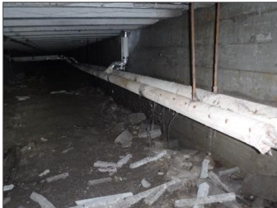
Asbestos-containing Aircell pipe insulation debris present on the dirt floor in tunnel.
