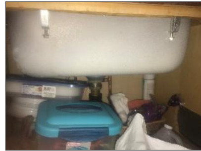
Non-asbestos grey / white sink mastic.
