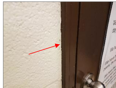
Asbestos-containing grey door frame caulking.
