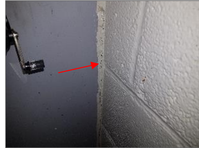
Asbestos-containing brown cementitious caulking around bookshelf Classroom 110.
