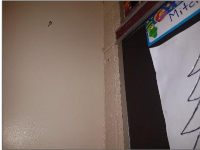
Non-asbestos white caulking on drywall in Classroom 107.
