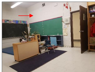
Photo 17 – Light beige paint on block wall containing elevated levels of lead.
