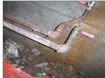
Asbestos-containing parging cement and Aircell debris on the tunnel dirt floor.
