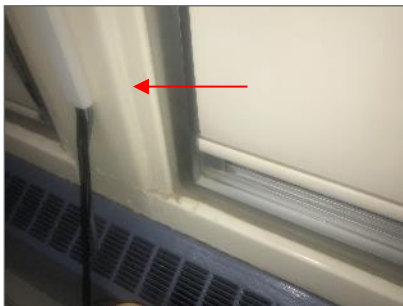
Asbestos-containing dark grey cementitious caulking between wood strips and exterior concrete wall column.
